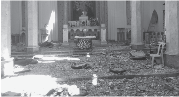
Rubble is scattered across what remains of Holy Spirit Church in Homs, Syria. It is one of several churches in Syria that have suffered severe damage from the ISIS bombings.
